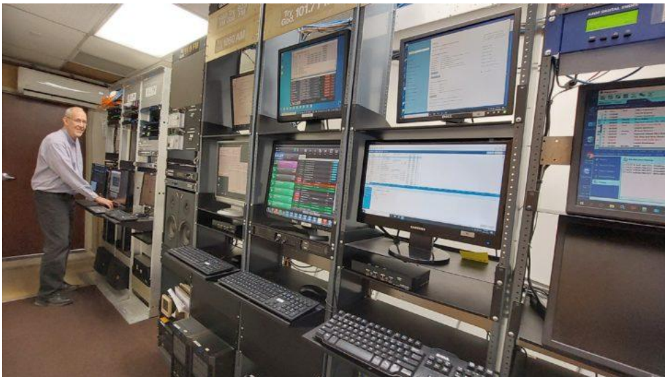
Bill Havas at work in the rack room, which includes hardware for the WheatNet and WideOrbit systems.
