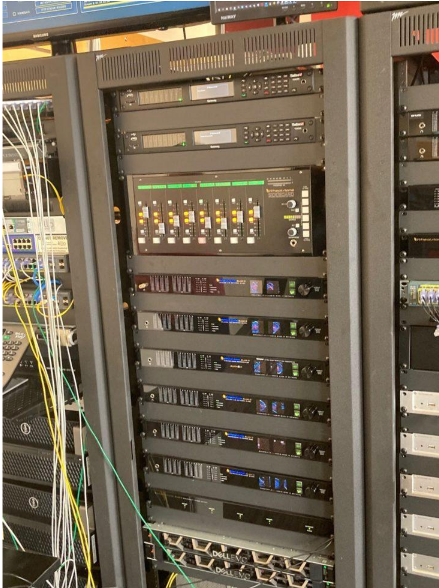
Tiline and WheatNet equipment is visible in the rack area
