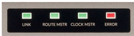
Figure 2-5 Mix Engine Front Panel Status LEDs
